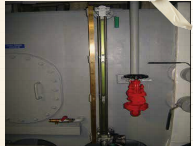
Fuel tank "Day Tank" with level indicator Day Tank
